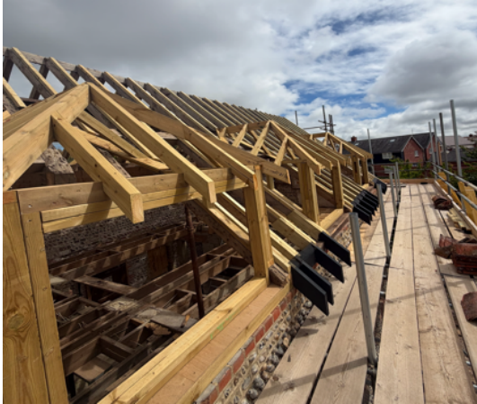
Plate 7: Stripped Southern Roof
