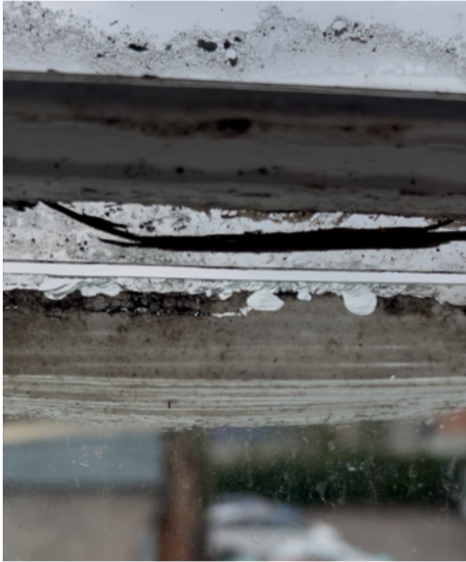
Pane partially detached with a pronounced gap between panes and edge chipping, indicating compromised stability
