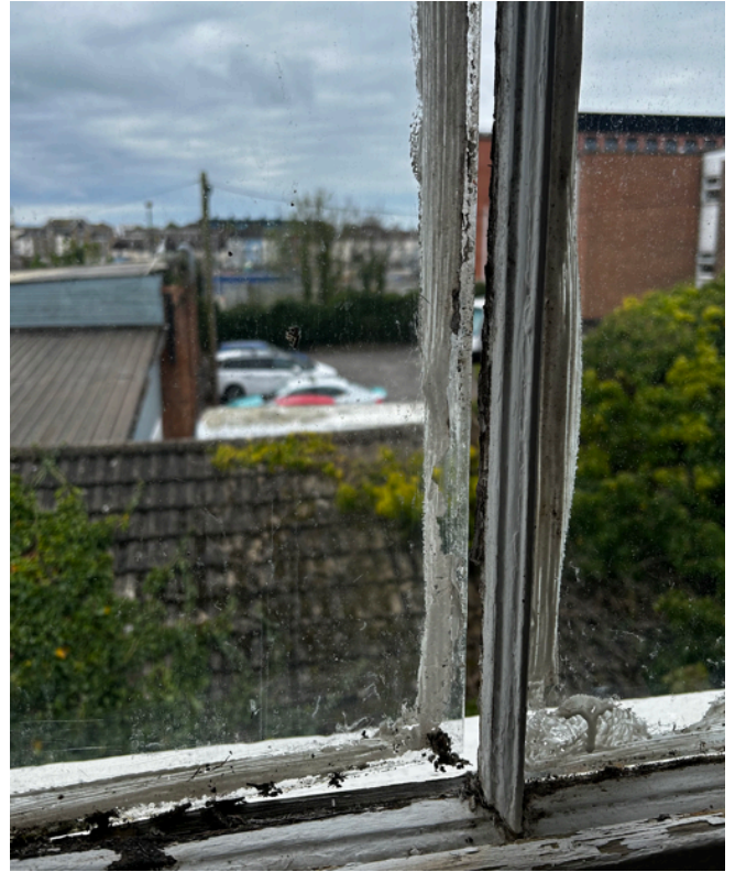
Failed putty and open joints allowing water ingress
