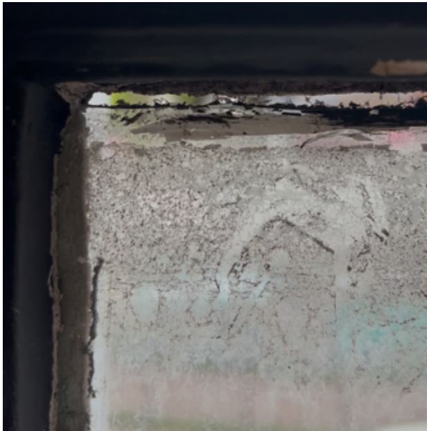
Loose pane with failed putty
