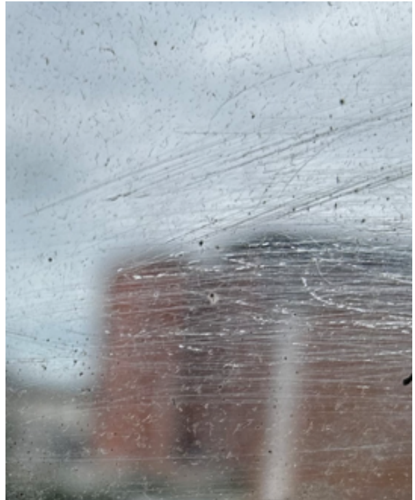
Pane showing significant scratching affecting visibility
