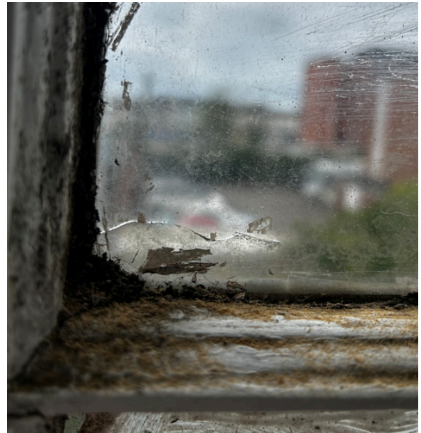
Crack across glazing pane compromising integrity
