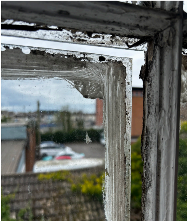
Pane displaced from frame with visible gap and movement. Presenting severe safety risk.
