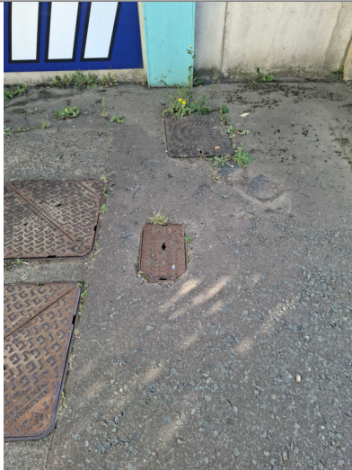
Other Site Photos: WASHOUT
