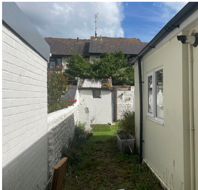
Narrow, shaded and damp outside space between the existing outrigger and neighbouring extension - note the much sunnier garden beyond.
