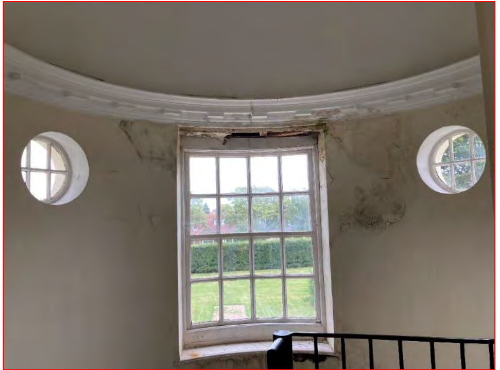
Plate 34 View of bullseye windows and sash window at first floor level (within eastern stairwell). This image dates from 2021. The evident moisture penetration to the plasterwork was subsequently dealt with as part of the school conversion with the plasterwork restored and redecorated.
