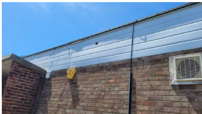
Left: Eastern aspect of B1 with hole in plastic fascia PRF visible.
