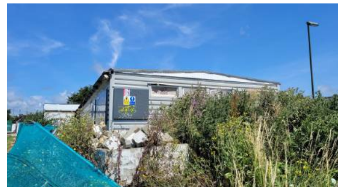
Right: Southern aspect of B2 with PRFs including the raised window flashing and gap besides drainpipe.
