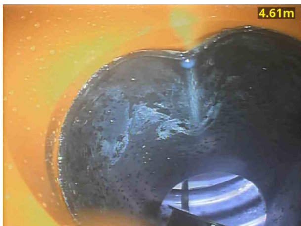
2_S16_Upstream_LINE 1.jpg, 00:00:22, 4.60 m Deformed sewer or drain, 10%, IN GULLY ENTRANCE
