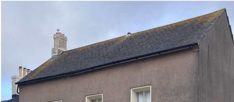
Existing roof slate with heavy build-up of lichen and moss.
