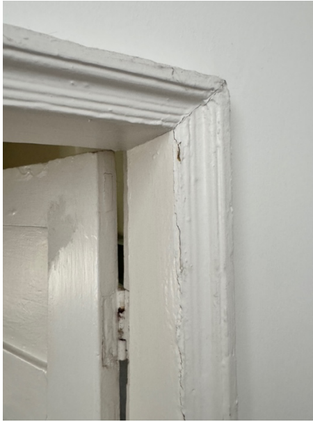
Existing architraves to first floor look to be original but in poor condition
