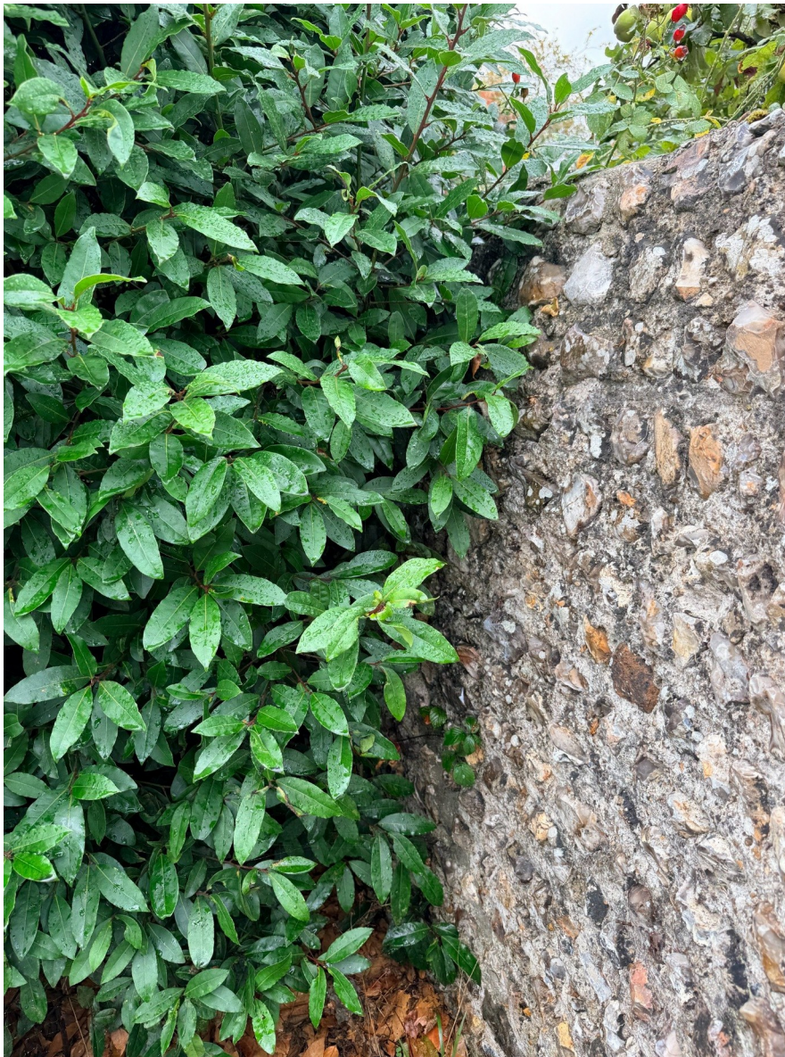
Photograph T3-A. Detail showing the Bay growth in very close proximity to the historic flint wall.
