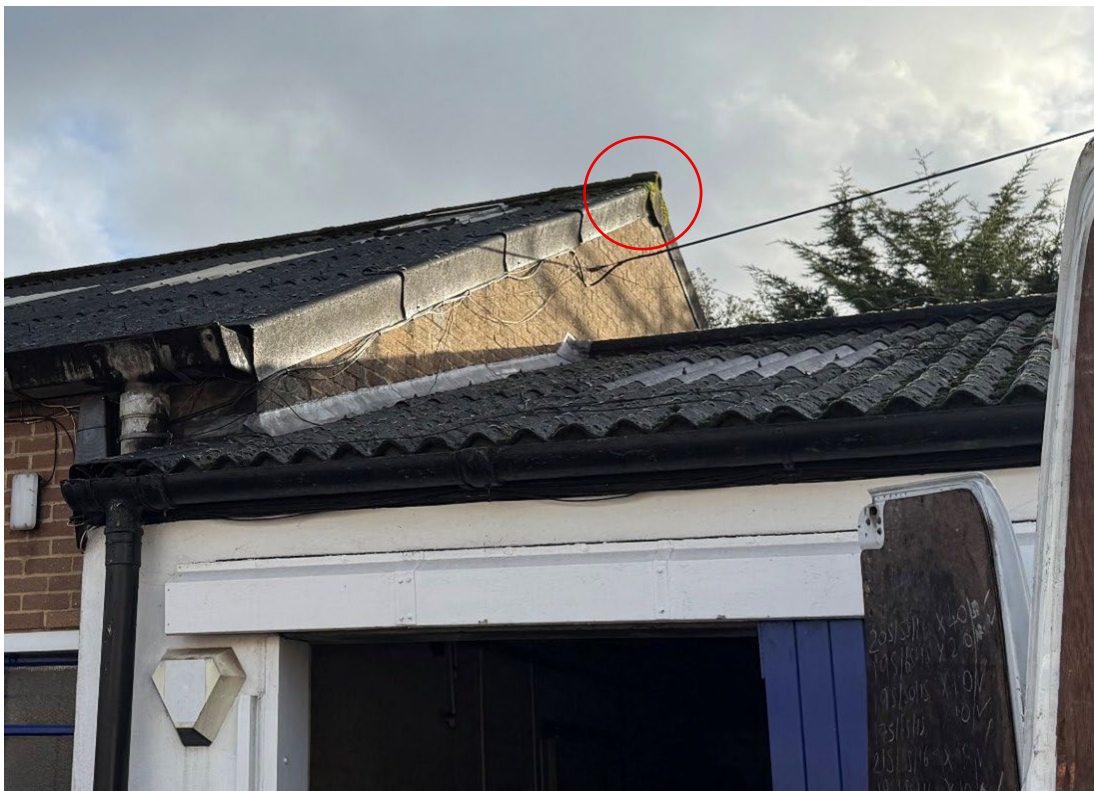
Photo 7: Building B3 has a corrugated sheet roof with a ridge capping. The capping is open at the eastern elevation gable end.
