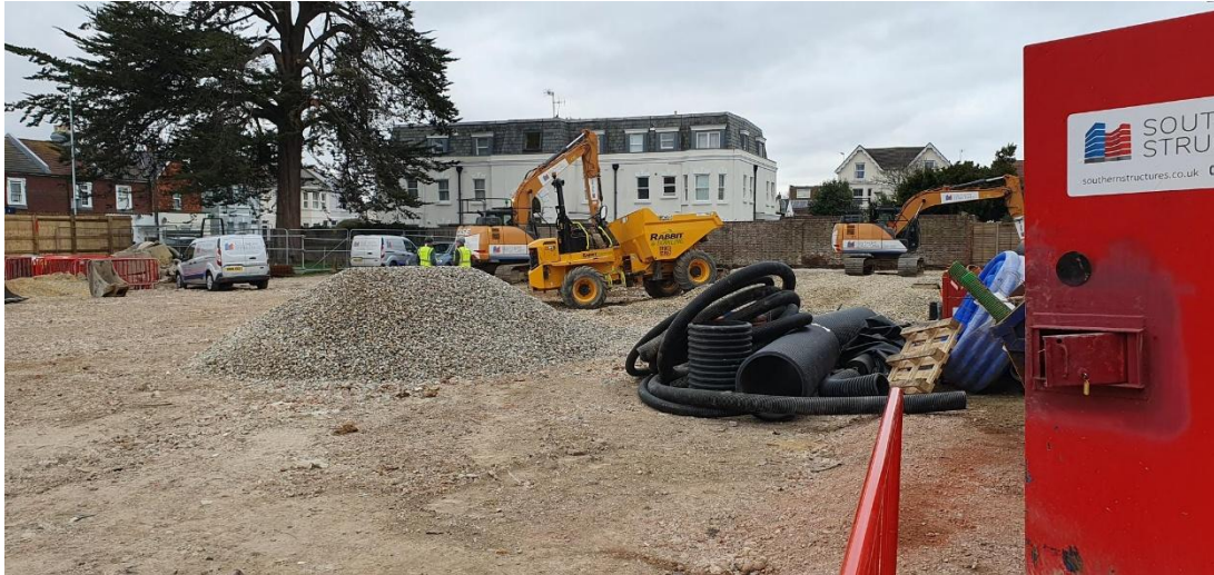
Voided Stone to rear car park
