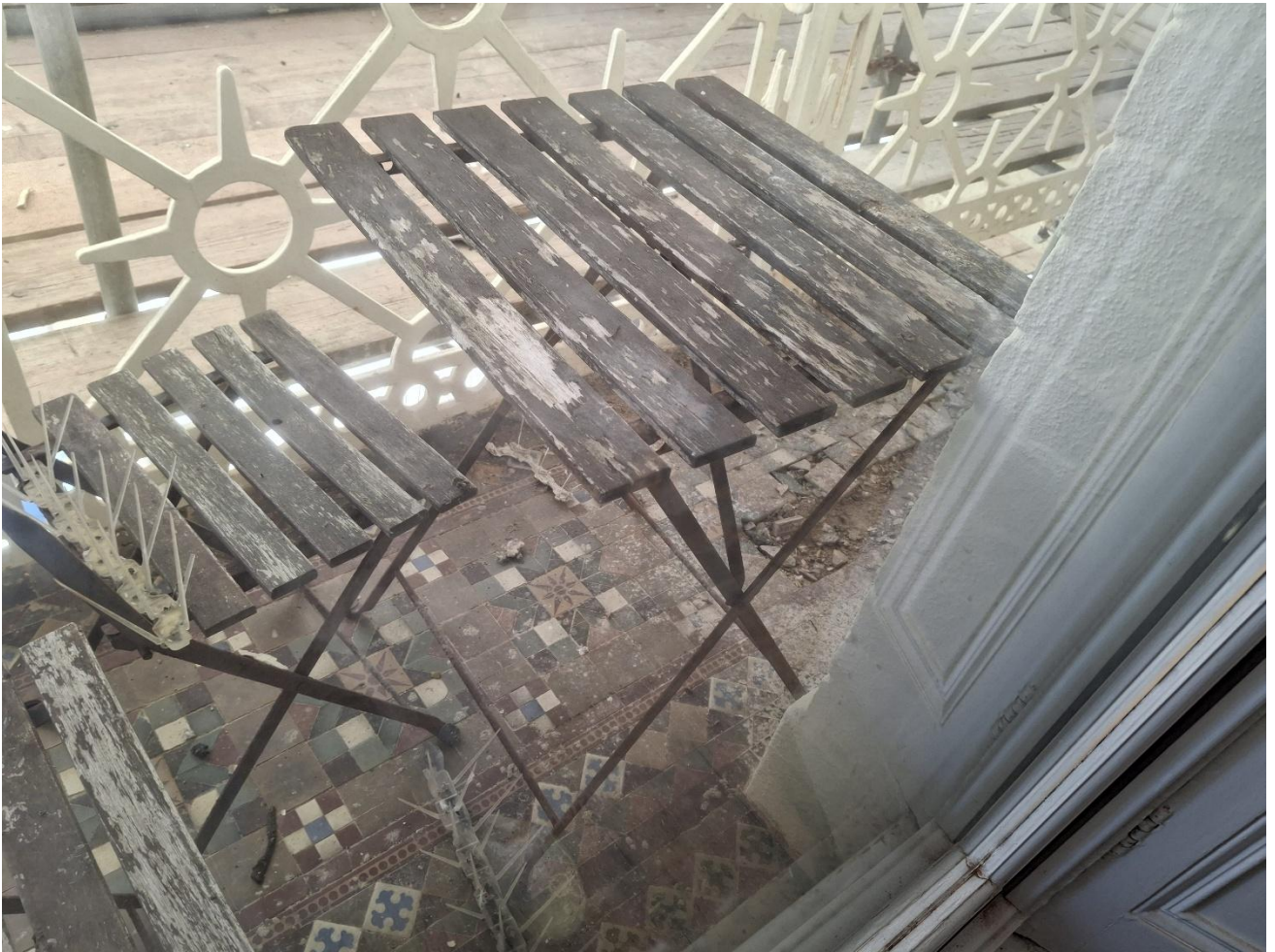
Figure 8: View of the balcony from the interior, showing damage to the tiles
