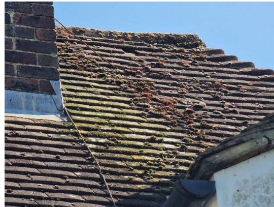
Figure 6: Missing tile on the western pitch towards the southern end.
