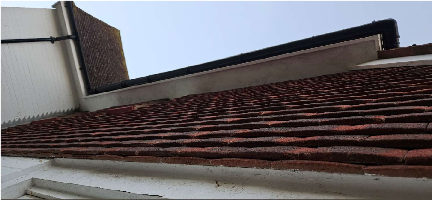
Photo 3 – Front section of hanging tiles demonstrating very tight fit with little bat roost potential
