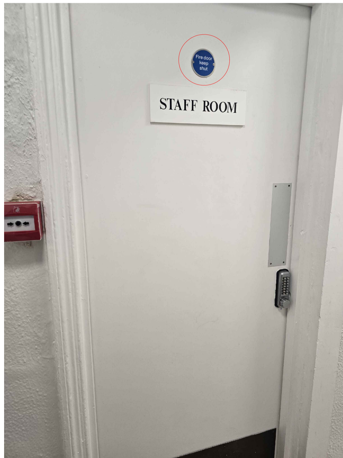
Existing door is already a fire door and there is no need to remove or replace it.
