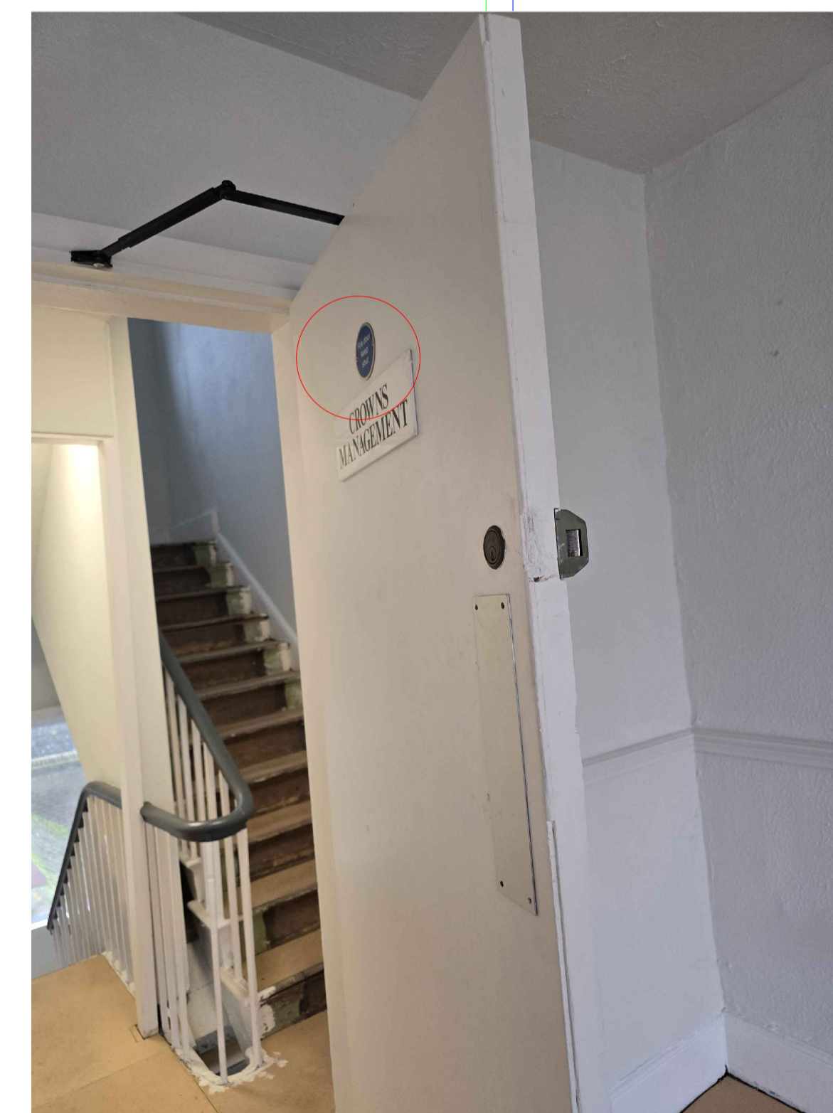
Existing door to be removed, and re-used in the proposed new door to living room. This is the only door proposed to be removed, however it will be re-used in the new location.
