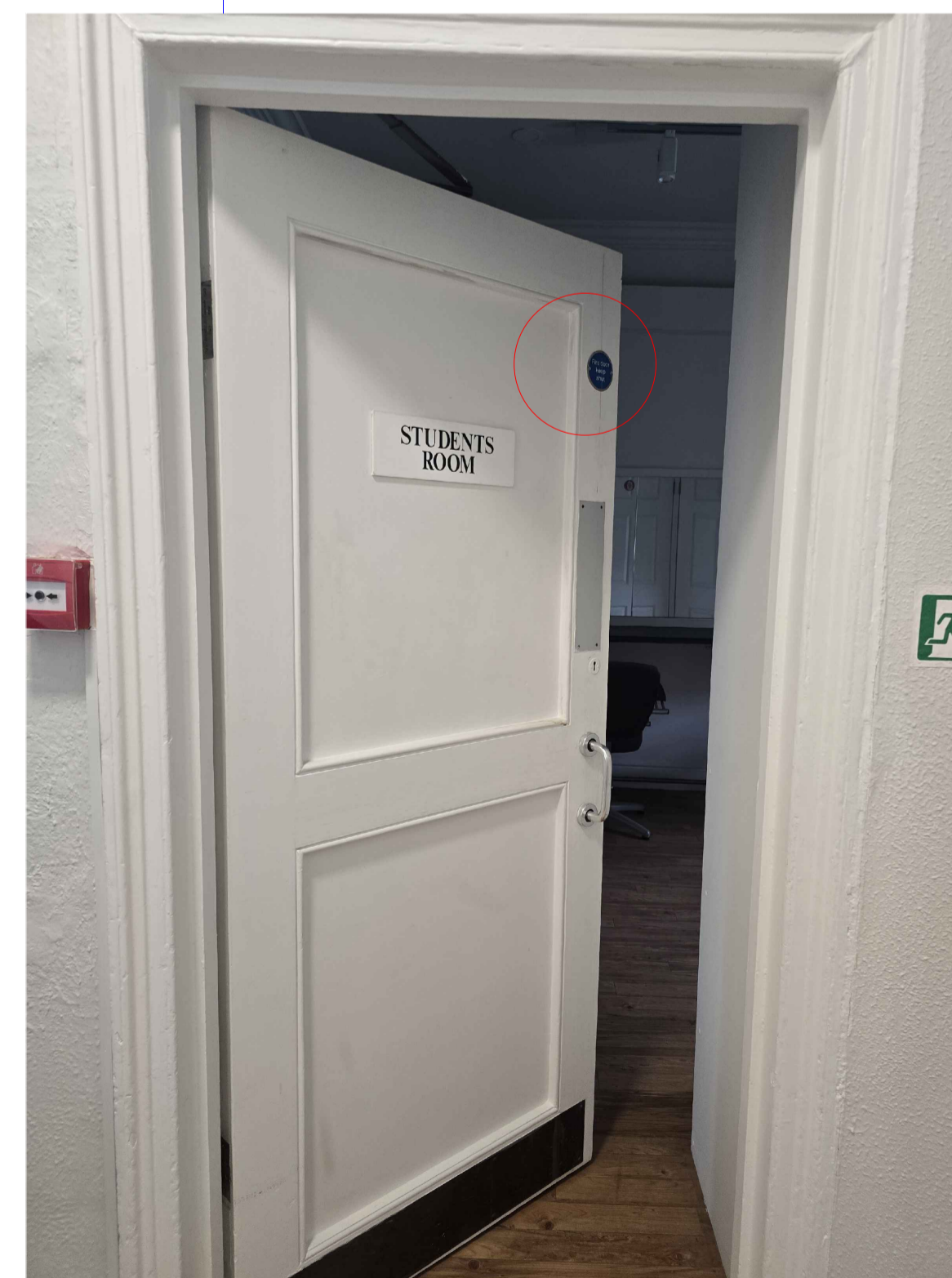
Existing door is already a fire door and there is no need to remove or replace it.
