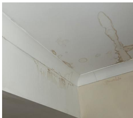
Figure 2: Example water damage to lower ground floor flats
