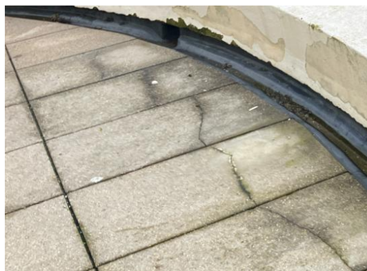
Figure 5: Cracking of existing screed
