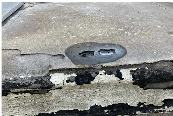
Figure 4: Typical example of asphalt condition
