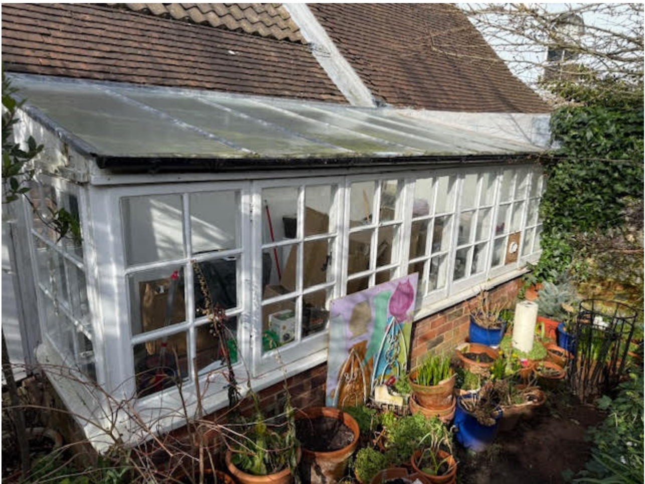
Fig.2 Existing Utility extension with glass roof, single skin damp walls
