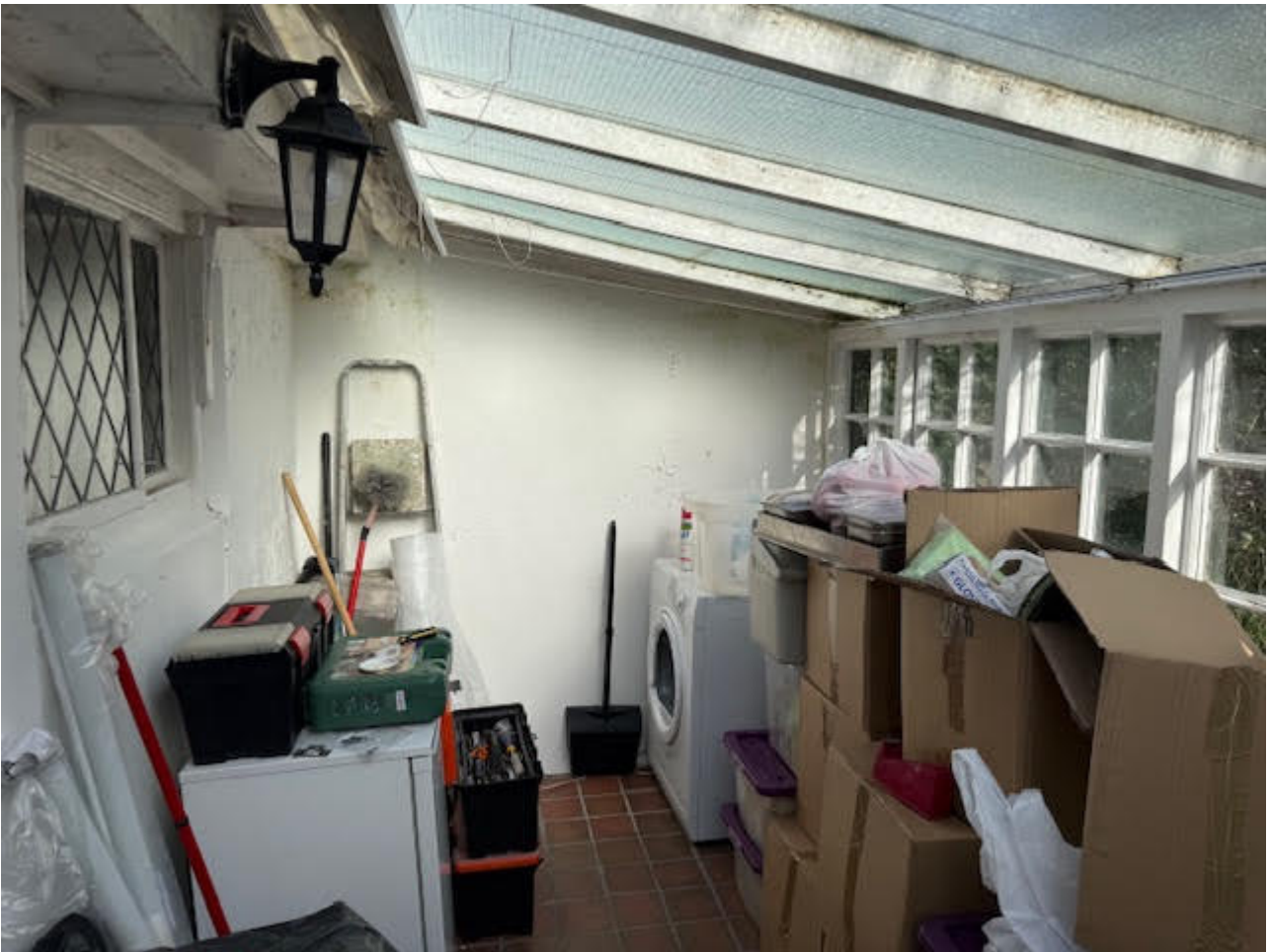
Fig 3. Existing utility extension showing damp walls. Sub-standard construction.
