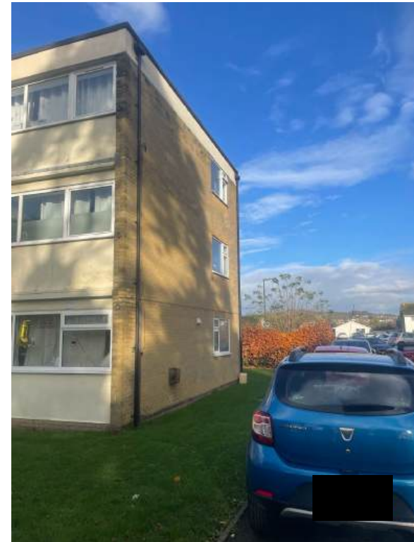
Plate 16 - guttering down western block of flats
