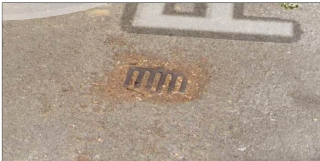
Figures 5.2 and 5.3 – Blocked existing drainage gulley
