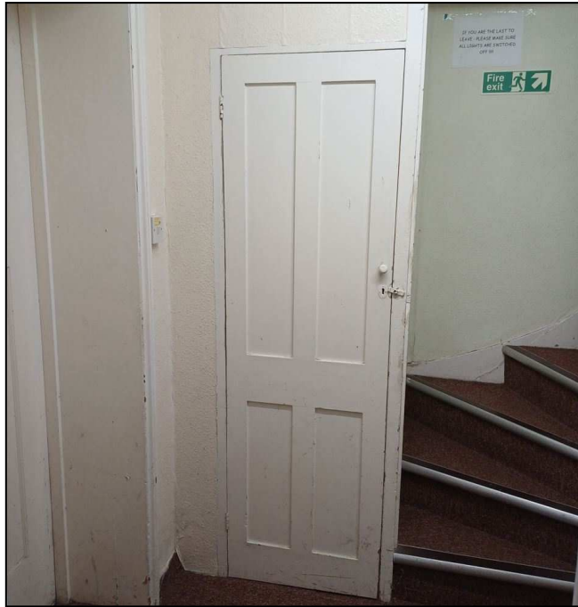
Door BD01 Basement Floor
