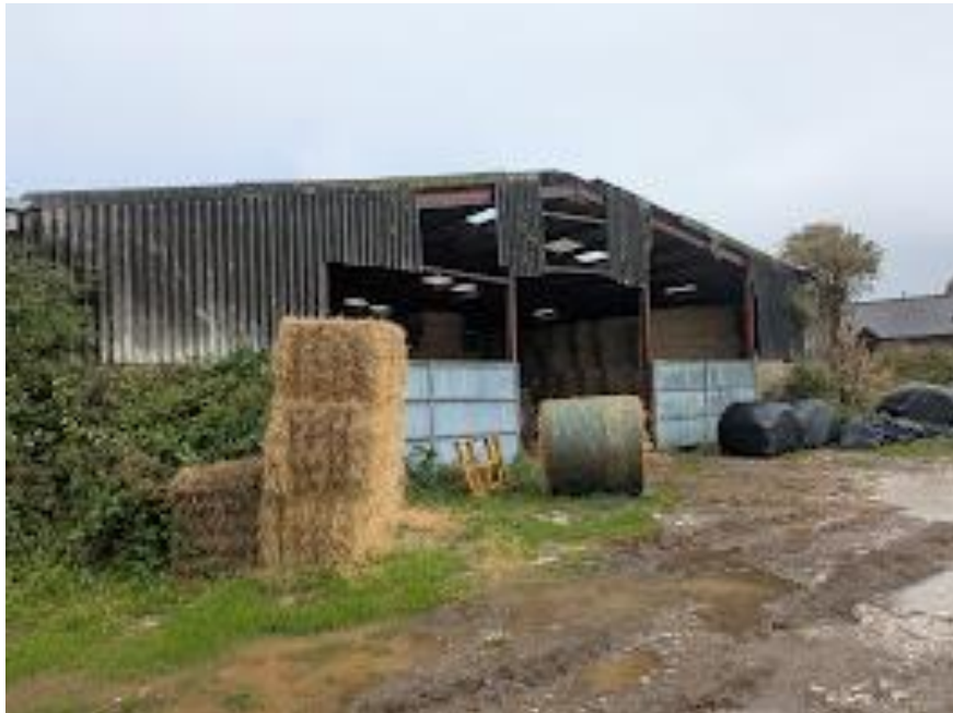
Photo 15. Damage to corrugated cement sheeting in the north-eastern barn.
