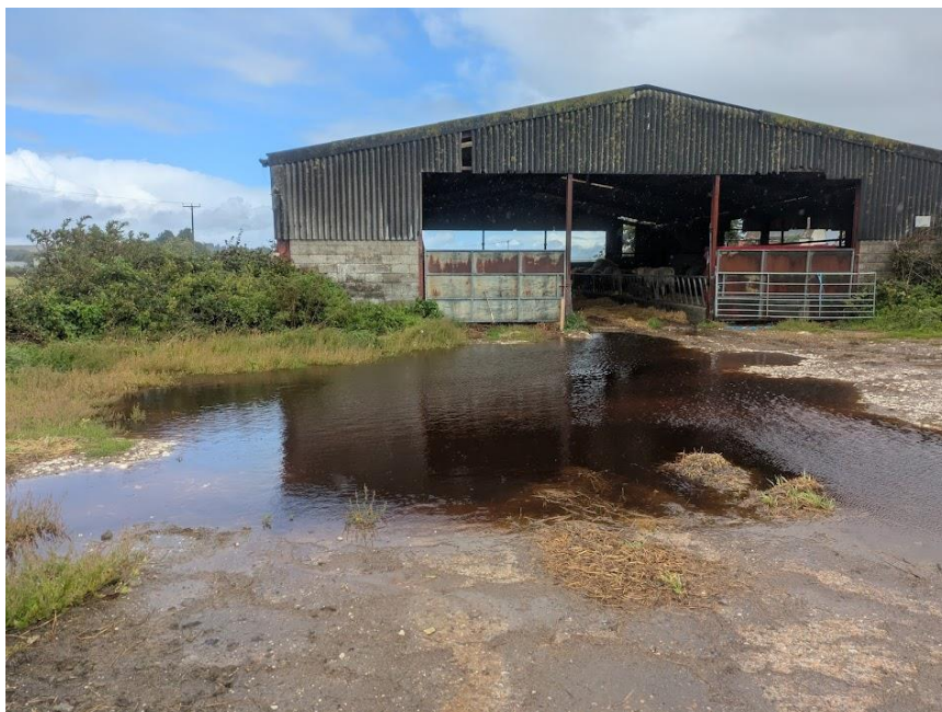
Photo 14. Surface water collecting in the centre of the Site, with leaching from manure stockpile/barns visible.
