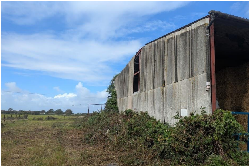
Photo 19. Damage to the southern barn.
