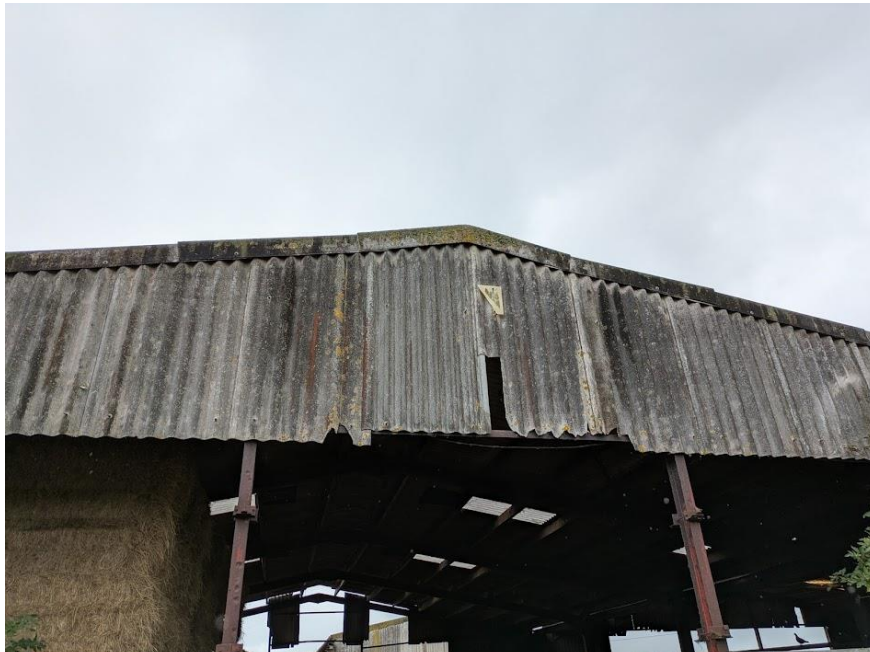
Photo 7. Corrugated cement/metal sheeting roof, with visible damage.
