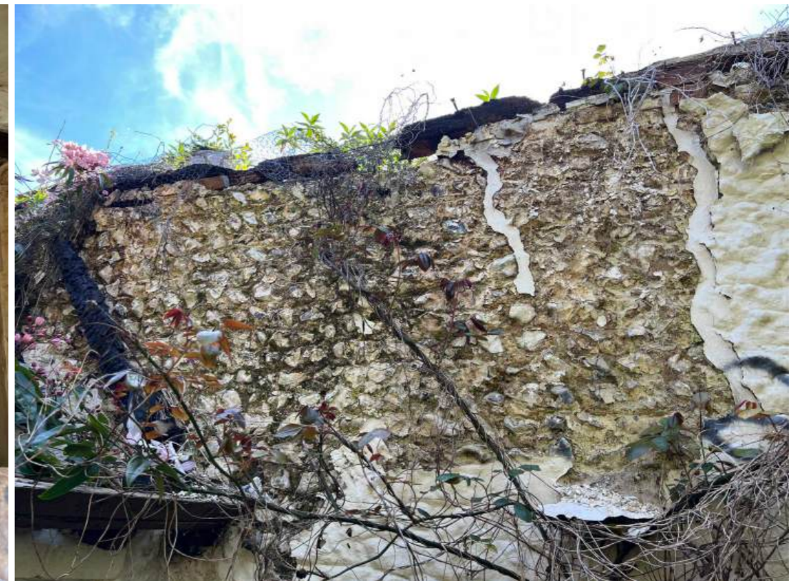
North elevation flint coursing revealed through the effects of weather, spring 2025.
