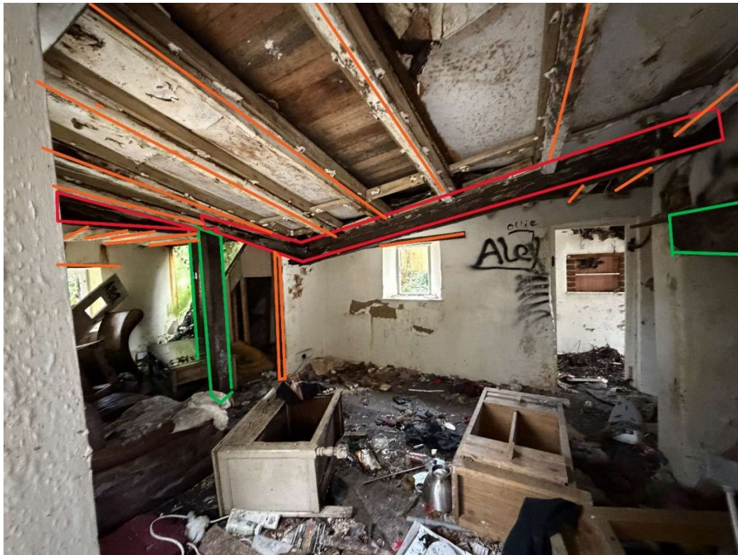
Figure 3. Internal ground floor structural timber elements to retain (green), review/repair (orange) or replace (red) (Jan '26 images).
