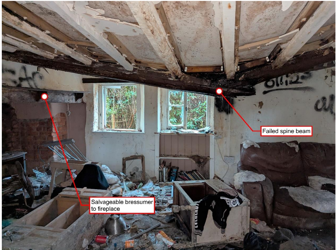
Photo 10 – Failed spine beam
