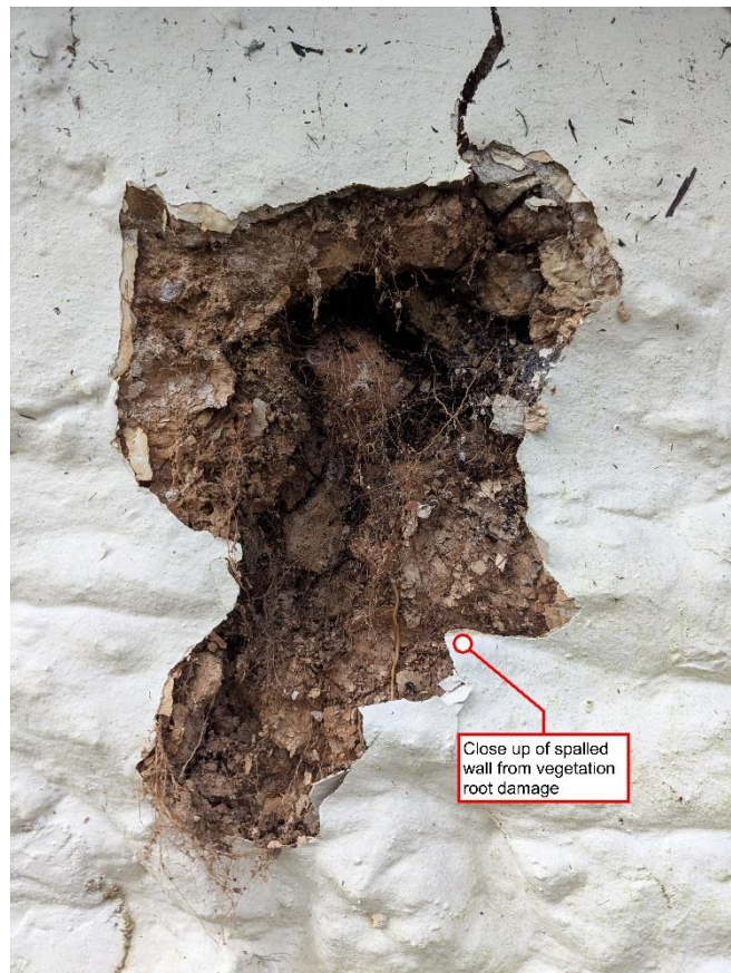
Photo 14 – Vegetation damage close-up
