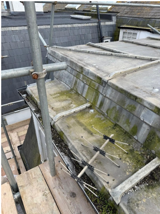
Flat roof showing multiple sheets and nailed seams.
