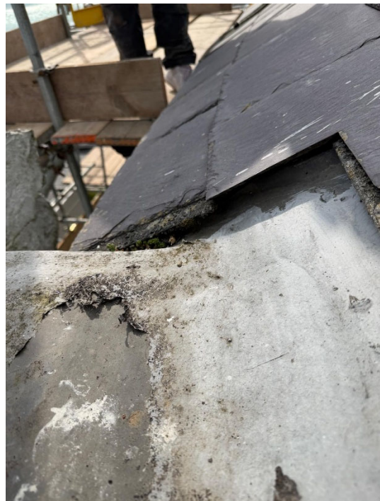
Example of failed flashing at roof junction.
