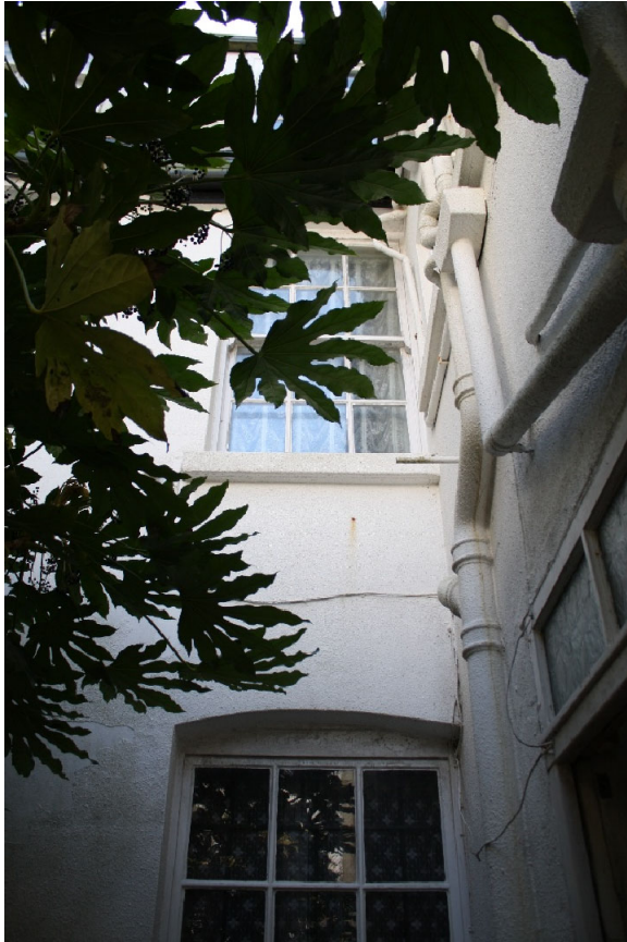
First floor W5 bottom – view obscured. To be overhauled.
