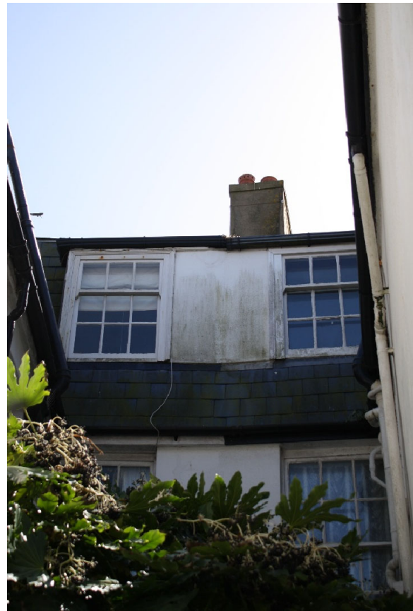
First floor W5 top – view obscured. Second floor W10 – to be overhauled.
