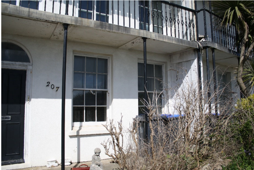
2no. W1 – to be overhauled.
