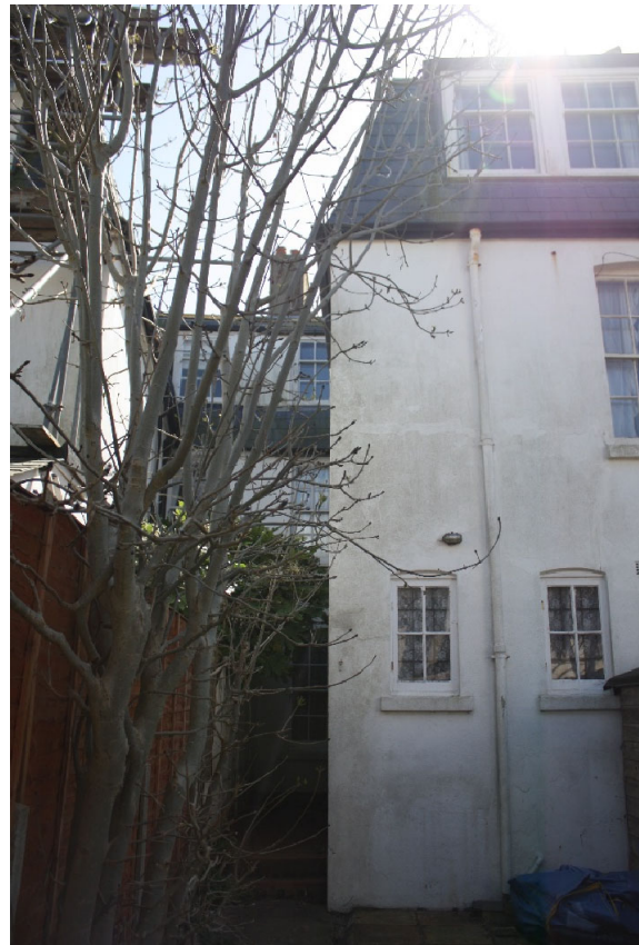
Ground floor 3no. W4 – to be replaced
