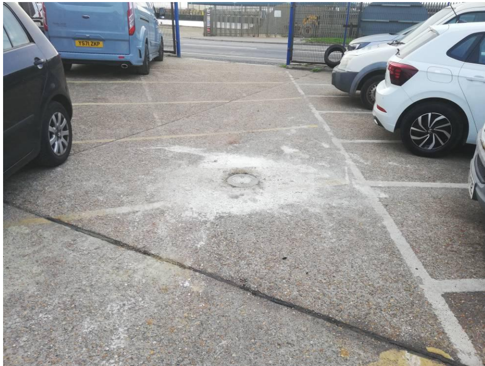
WS5 MONITORING WELL PROTECTED BY FLUSH COVER
