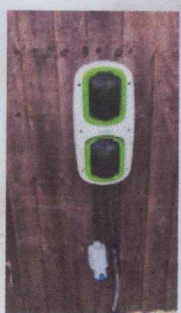
Electric vehicle charging point
