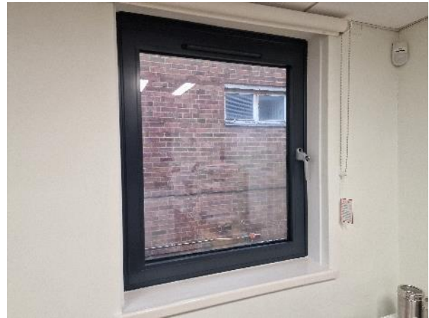
22. Replacement aluminium framed window to rear
