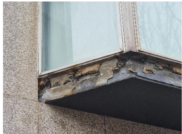
4. Defective cladding to bay windows
