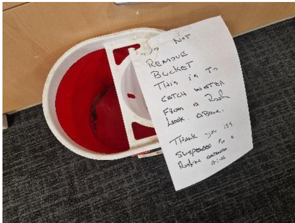
17. Evidence of water ingress internally
