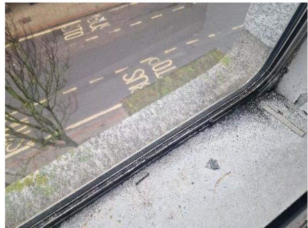
8. Degraded sealant to window frames
