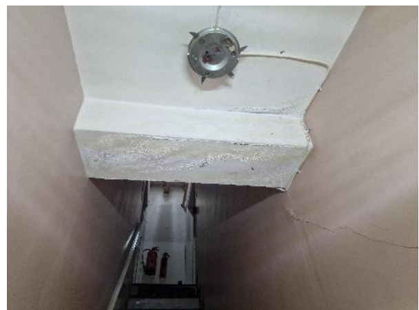
10. Evidence of moisture ingress internally
