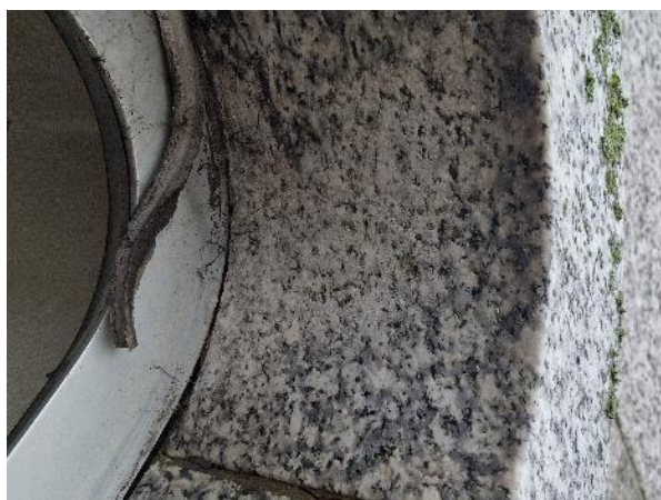
9. Degraded sealant to window frames
