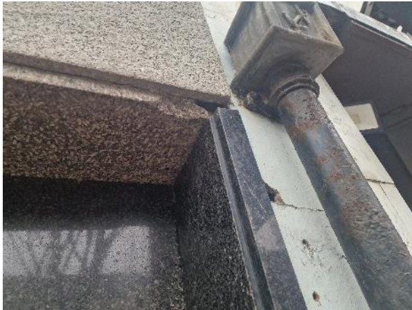
5. Damaged cladding at ground level
