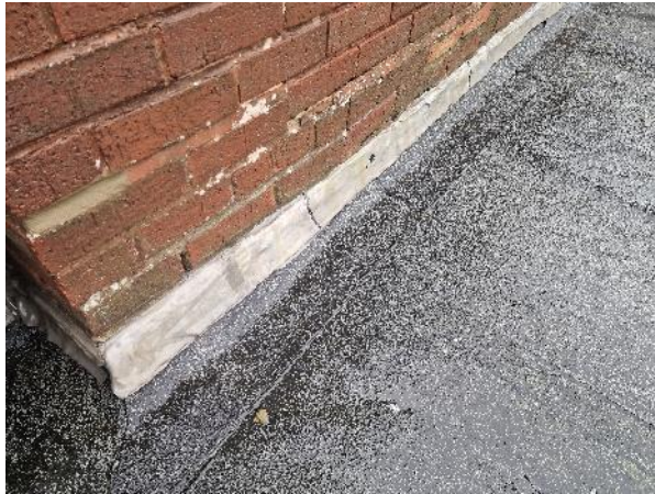
15. Poor flashing detail to lower flat roof
