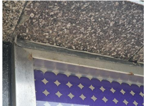
6. Degraded sealant to window frames
