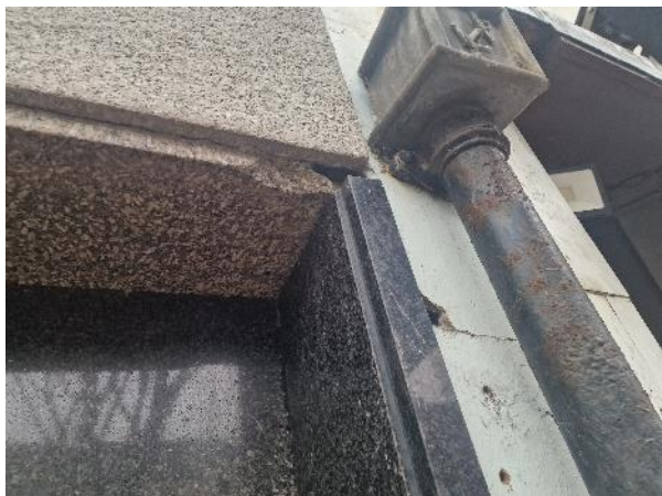
5. Damaged cladding at ground level
