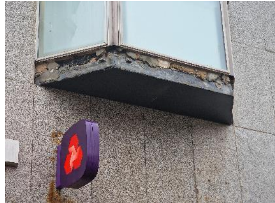
Photograph E – Removed cladding to foot of bay window
