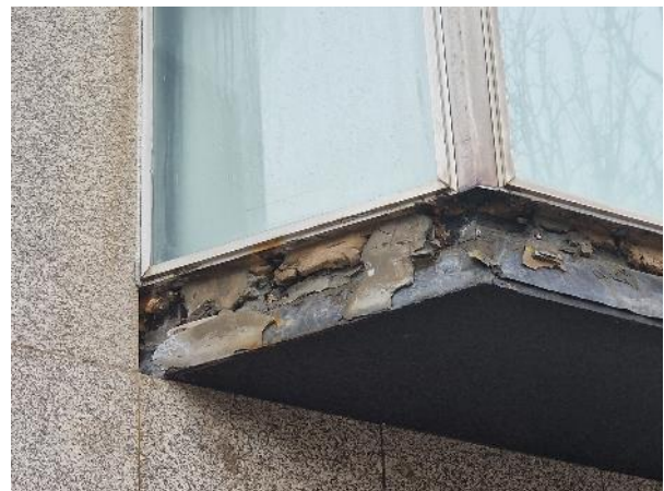
4. Defective cladding to bay windows
