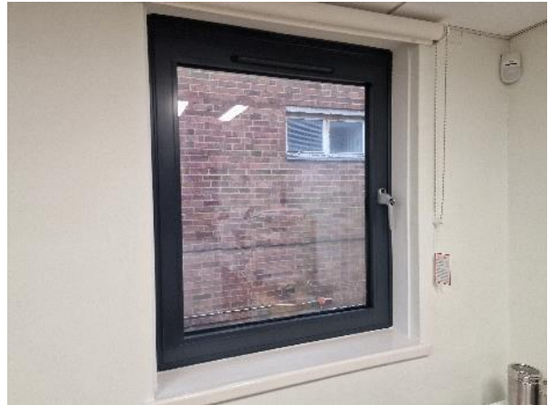
22. Replacement aluminium framed window to rear
