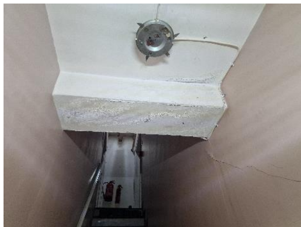
10. Evidence of moisture ingress internally
