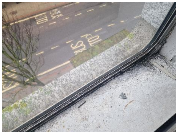
8. Degraded sealant to window frames
