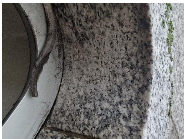
9. Degraded sealant to window frames
