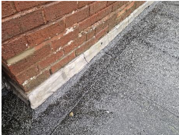
15. Poor flashing detail to lower flat roof
