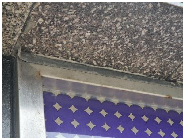
6. Degraded sealant to window frames
