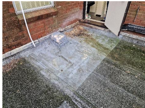
18. Poor patch repair to lower flat roof – Roof 3
