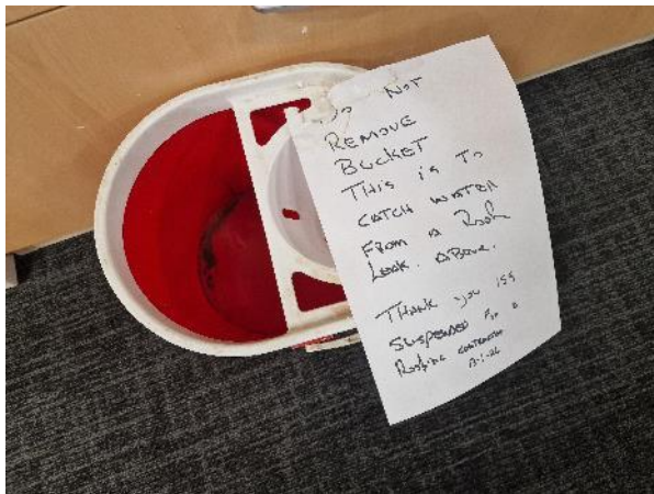
17. Evidence of water ingress internally
