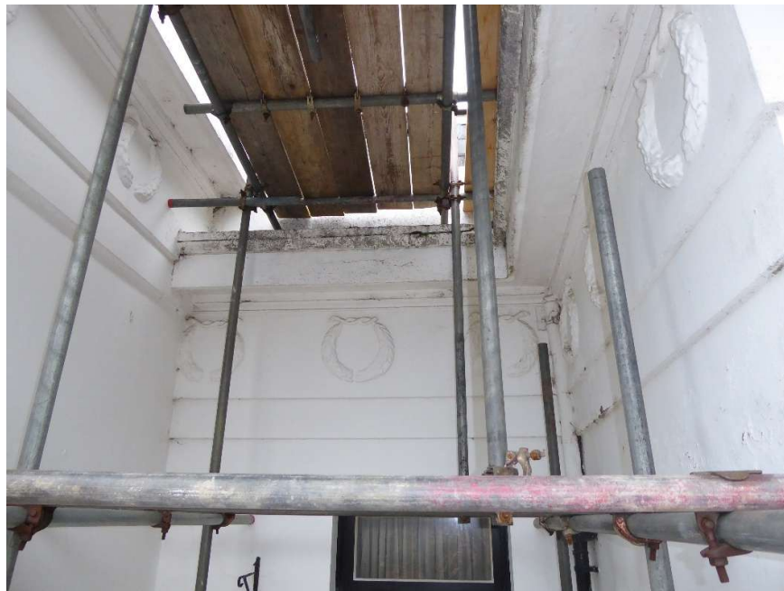
Fig 2. Front elevation showing the existing rainwater goods below second floor.
