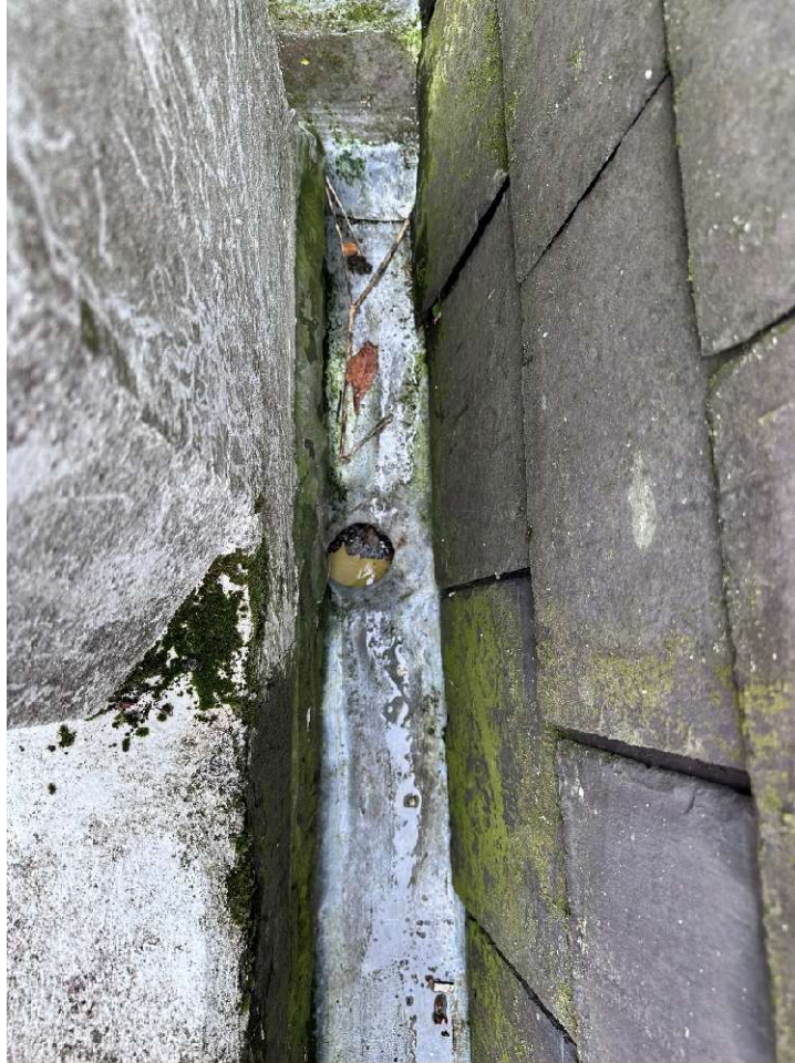
Fig 3. Existing blocked gully. Inaccessible without scaffolding to front elevation.
