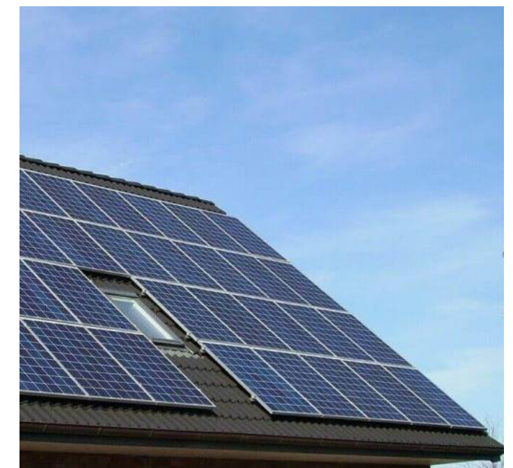
PV's on Roofs
