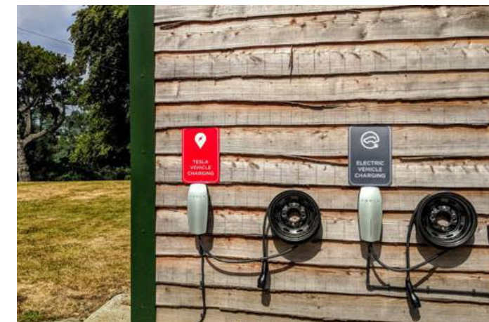
Electric Vehicle Charging Points
