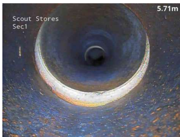
12, 00:01:28, 5.90 m Joint displaced, medium
