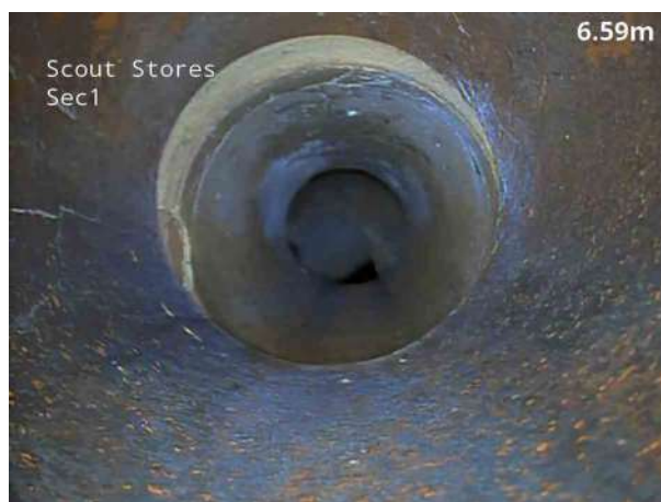
14, 00:01:37, 6.80 m Joint displaced, medium
