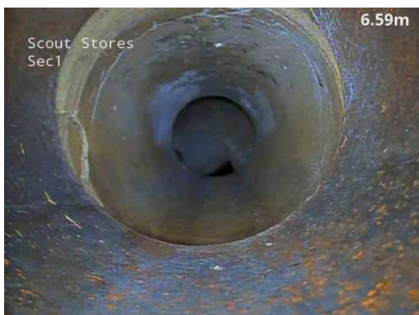
13, 00:01:35, 6.80 m Fracture, circumferential at joint from 8 o'clock to 4 o'clock
