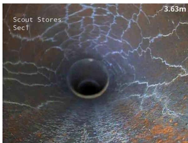
8, 00:00:57, 3.60 m Cracks, multiple from 8 o'clock to 4 o'clock, change
