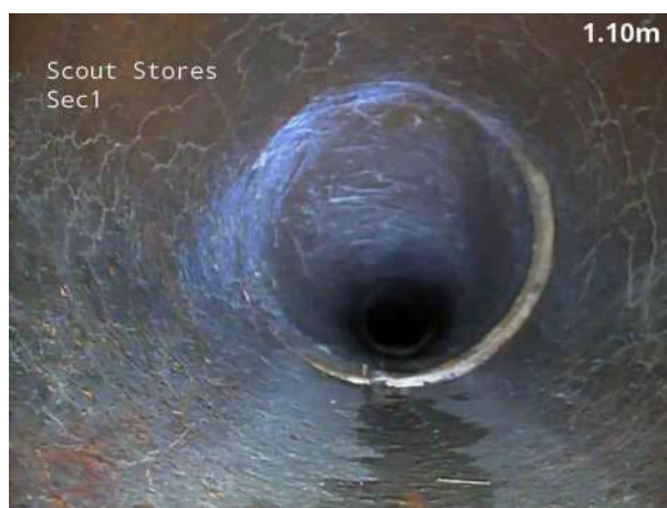
4, 00:00:11, 0.90 m Cracks, multiple from 8 o'clock to 4 o'clock, start
