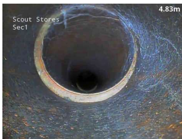
10, 00:01:21, 5.00 m Joint displaced, medium
