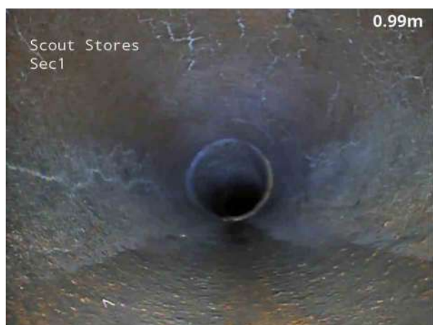
3, 00:00:11, 0.90 m Cracks, multiple from 8 o'clock to 4 o'clock, start
