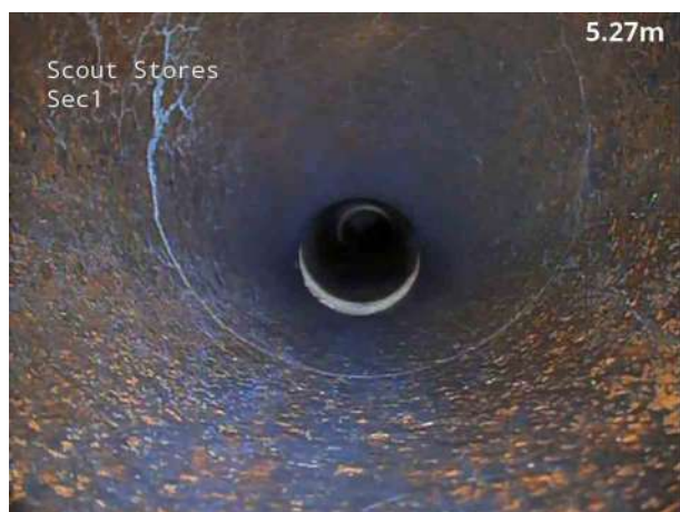
11, 00:01:25, 5.40 m Fracture, circumferential from 12 o'clock to 12 o'clock
