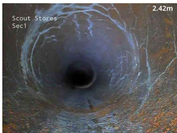
7, 00:00:43, 2.60 m Cracks, multiple from 12 o'clock to 12 o'clock, change
