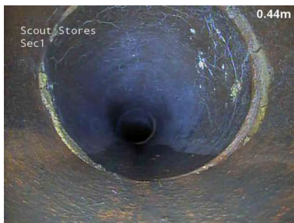
2, 00:00:08, 0.70 m Fractures, multiple at joint from 12 o'clock to 12 o'clock
