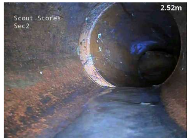
4, 00:00:31, 2.70 m Joint displaced, medium
