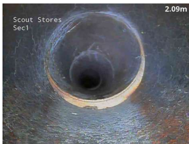
6, 00:00:31, 2.30 m Joint displaced, medium
