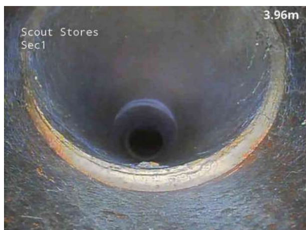
9, 00:01:12, 4.10 m Joint displaced, medium
