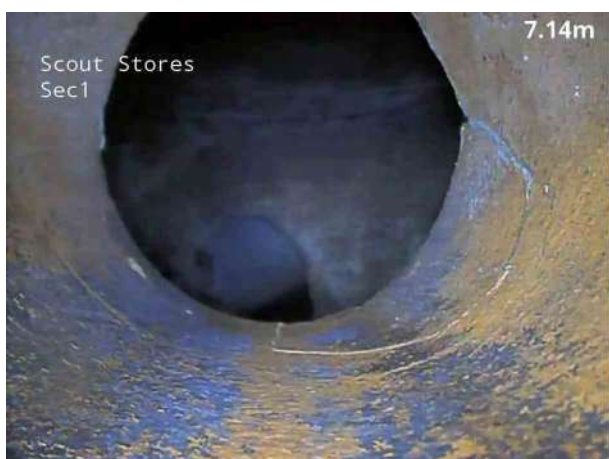
15, 00:01:43, 7.30 m Fracture, circumferential at joint from 3 o'clock to 9 o'clock
