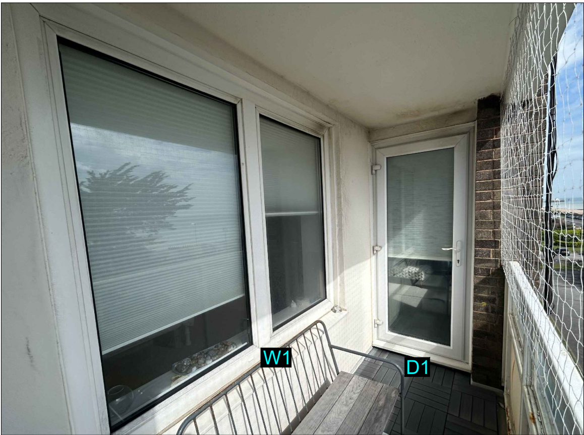
Photo Showing W1 & D1 on Balcony
