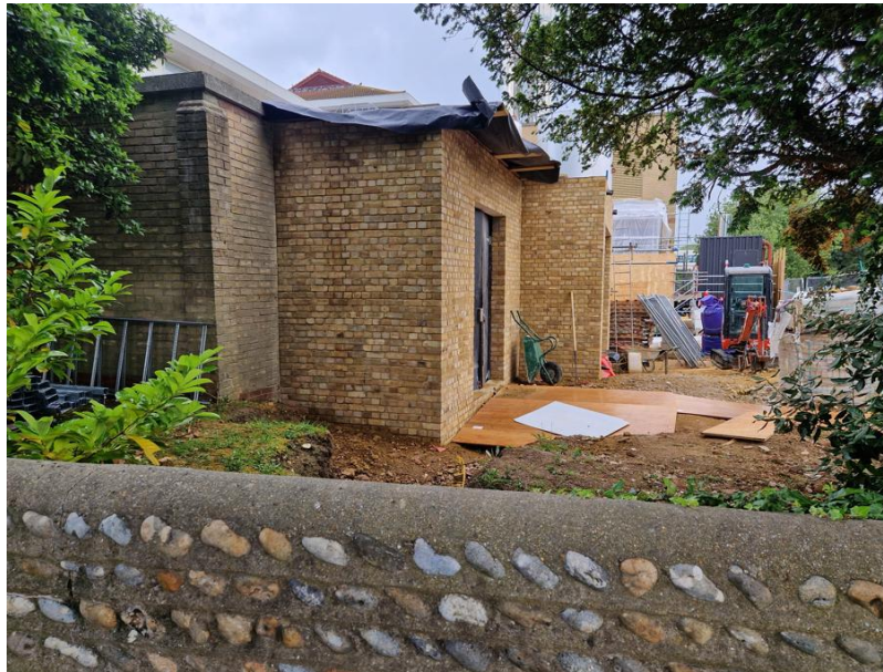
Figure 1: Amended Carpenter's Store and Transformer
