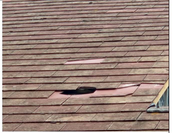
Photo 6: Example PRF – Damaged Roof Tile
