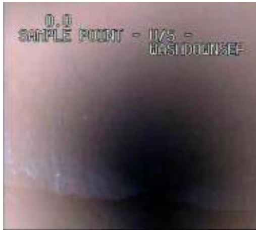
daac1b15-af8b-4760-831f-db02d498f400.png, 00:00:00, 0.00 m Start node, manhole, reference: sample poi
