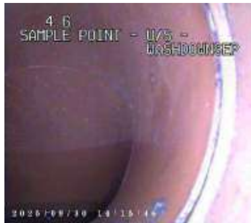
b06cba7f-5b36-425e-927f-b764aab2631a.png, 00:00:14, 4.60 m Finish node, oil separator, reference: washdownse
