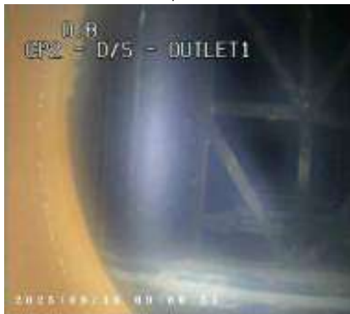
407488b1-cd58-4dcb-8f39-c59ea26d6a64.png, 00:00:18, 0.80 m Finish node, major connection without manhole, reference:
