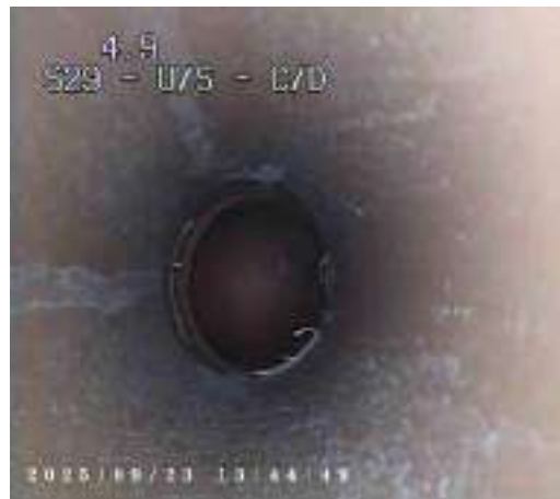
d3ecf7f5-2239-45f3-86d4-3b355595c19b_1.png, 00:00:21, 4.90 m Finish node, gully, reference: S29 CD
