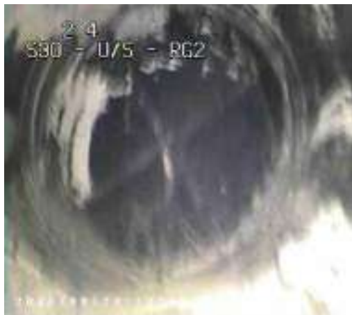
c108f169-65fd-4ba5-b04a-5ab6b7821191.png, 00:00:09, 2.40 m Finish node, manhole, reference: S30 rg2
