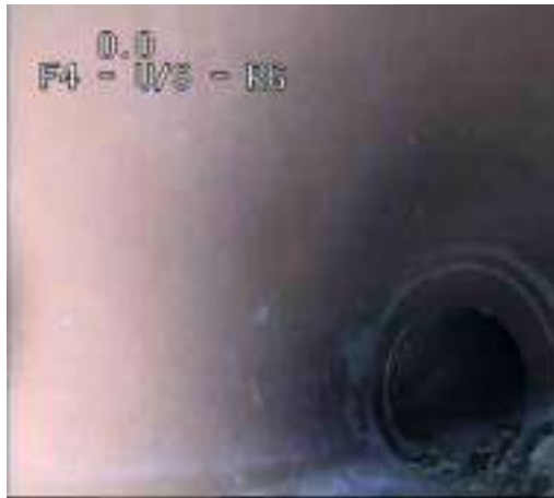
422db9b2-f356-4495-84a0-4c051dac8c5e.png, 00:00:01, 0.00 m Start node, inspection chamber, reference: F4
