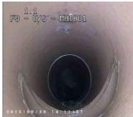
1c14b2c0-7be9-4dd5-9555-62820d6d5b08.png, 00:00:09, 1.10 m Finish node, manhole, reference: MH1801, back drop
