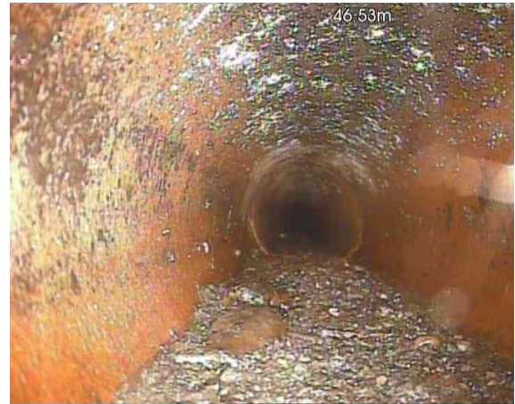
2, 00:02:39, 44.50 m Settled deposits, fine, 15% cross-sectional area loss
