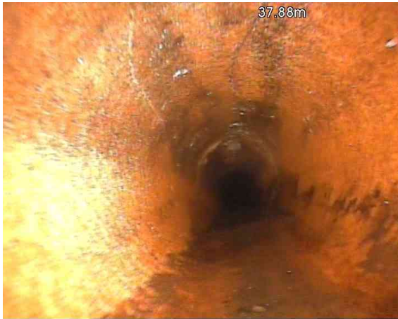
1, 00:02:31, 37.60 m Broken pipe from 12 o'clock to 5 o'clock
