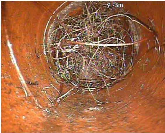
1, 00:00:39, 9.20 m Roots, mass, 80% cross-sectional area loss
