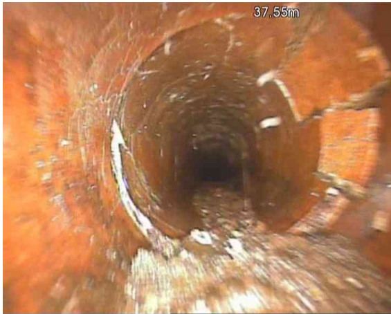
1, 00:01:34, 37.50 m Broken pipe from 12 o'clock to 4 o'clock
