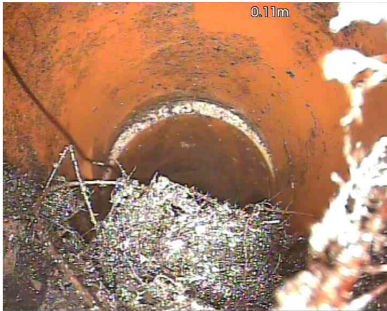
1, 00:00:11, 0.20 m Roots, mass, 15% cross-sectional area loss
