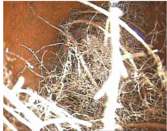
2, 00:00:32, 8.60 m Roots, mass, 75% cross-sectional area loss
