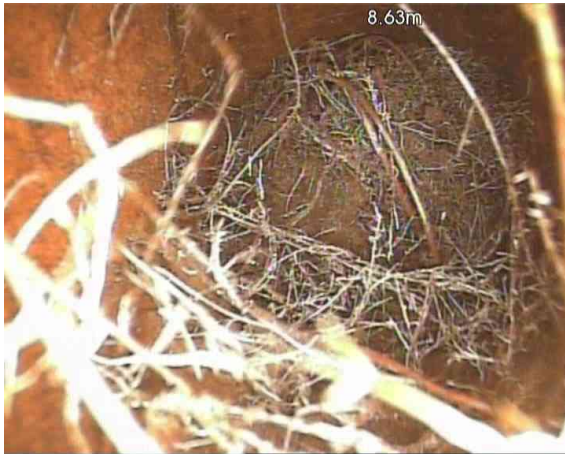
1, 00:00:32, 8.60 m Roots, mass, 75% cross-sectional area loss
