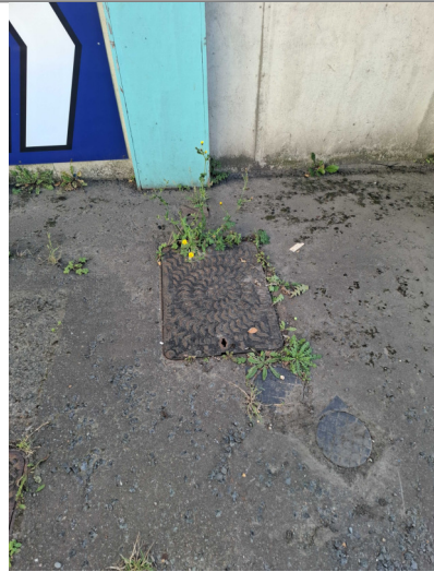
Other Site Photos: MAINS WATER LINE
