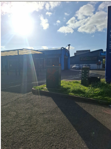
Other Site Photos: PUMP STATION PANEL
