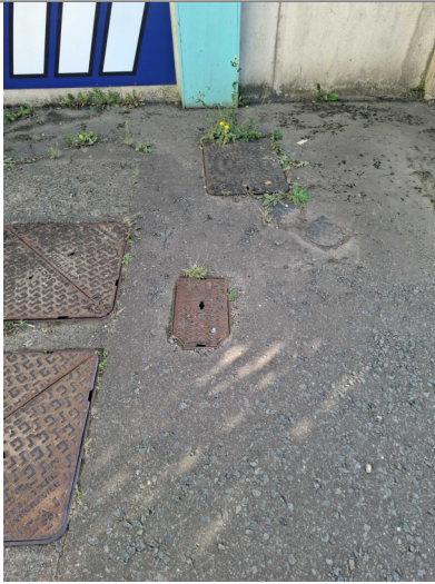
Other Site Photos: WASHOUT
