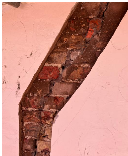
Figure 4: Cracking to curved bay – sheared brickwork
