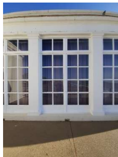
Fig 11: Typical Denton Lounge screen
