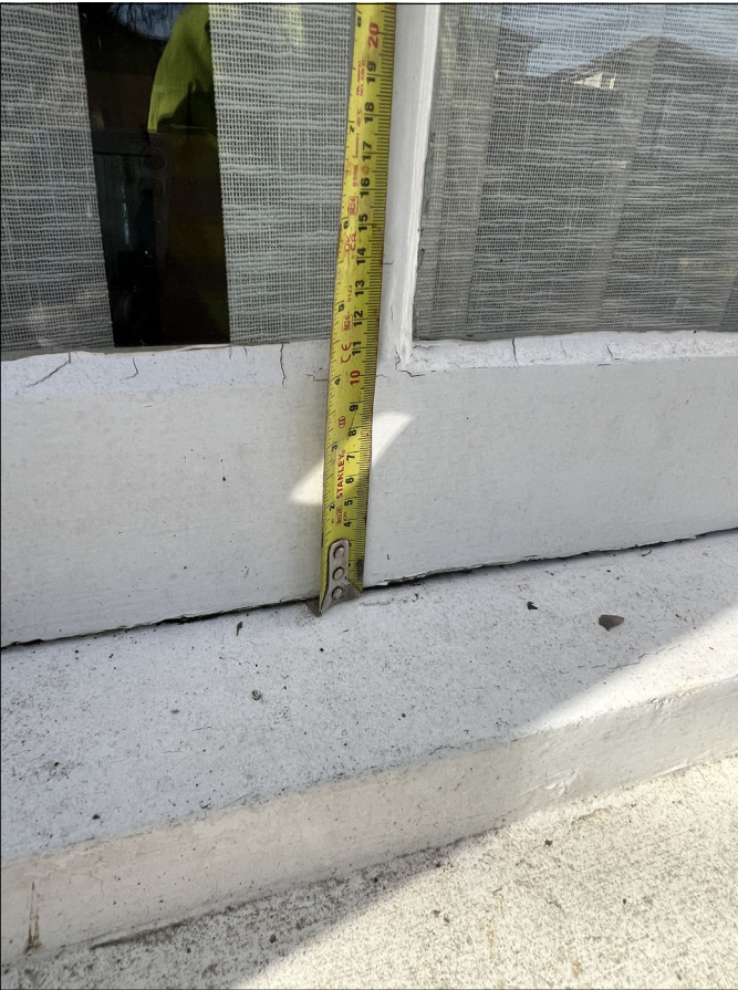
Photo of existing bottom rail - NTS
