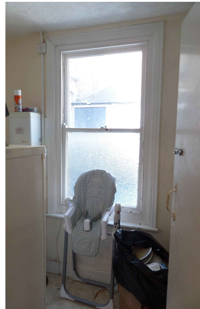
Internal view of outrigger - Refer to P019 for replacement
