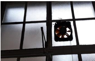
Female WC. FM to address window opening mechanism. Ease to allow closure. FM to replace damaged extract fan.
