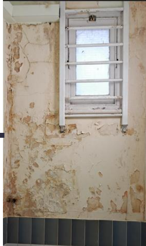
Dampness on WC wall face.. Wall overlooks Roof 4.
