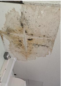
Damp ingress due to M&E noted and is currently being remedied by FM.
