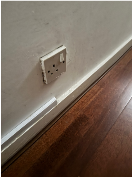
Existing non-original skirtings
