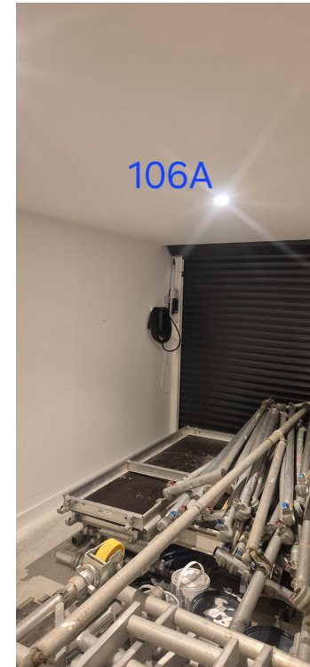
EV charger to No 106a (Plot 4)
