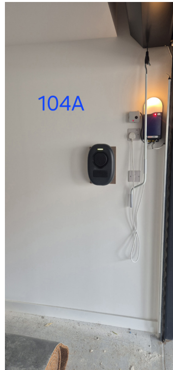
EV charger to No 104a (Plot 2)
