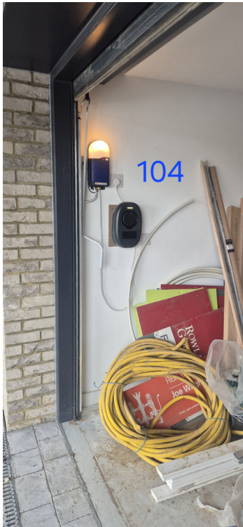
EV charger to No 104 (Plot 1)
