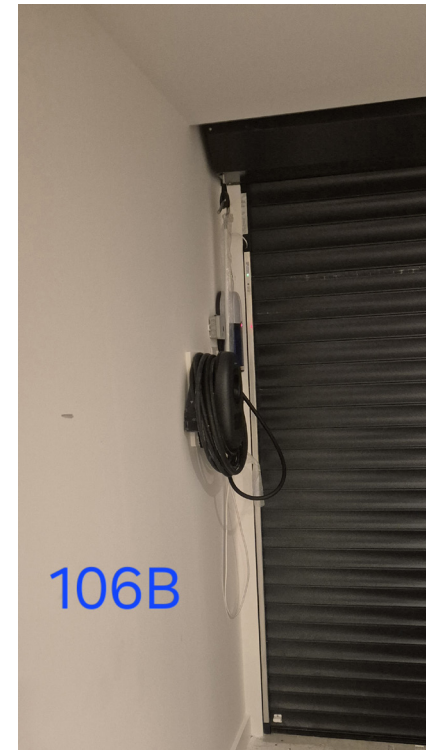
EV charger to No 106b (Plot 5)
