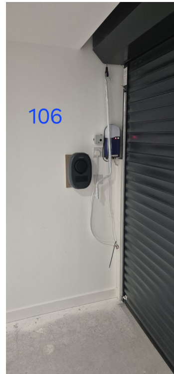
EV charger to No 106 (Plot 3)
